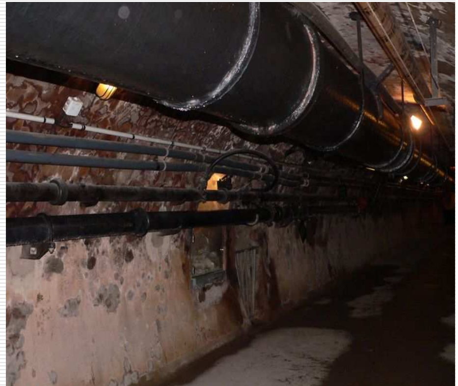
Kanalisation in Paris
